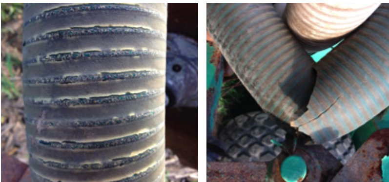
PVC Hose cracking due to UV exposure
