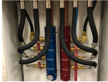
1-1/2" Manifold Assemblies Mounted in a Control Cabinet with Brass Ball Valves and Custom Hose Assemblies
