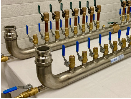
Large Supply and Return Manifold Assemblies with Pipe Extensions on Return Manifold for Non-Contact Flowmeters for Laser Cooling Application
