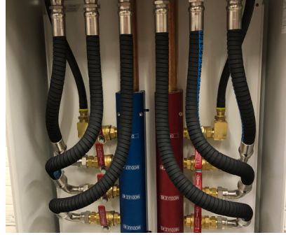
1 1/2" Aluminum Manifold Assemblies Mounted in a Control Cabinet with Brass Ball Valves and Custom Hose Assemblies
