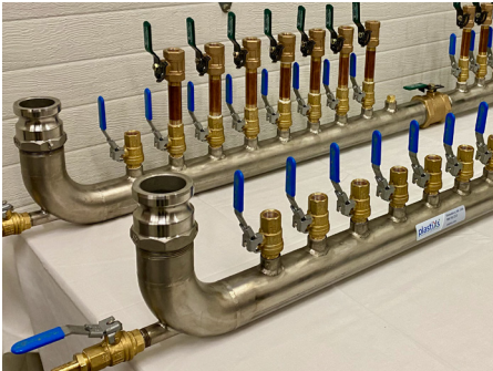
Large Supply and Return Manifold Assemblies with Pipe Extensions on Return Manifold for Non-Contact Flowmeters for Laser Cooling Application
